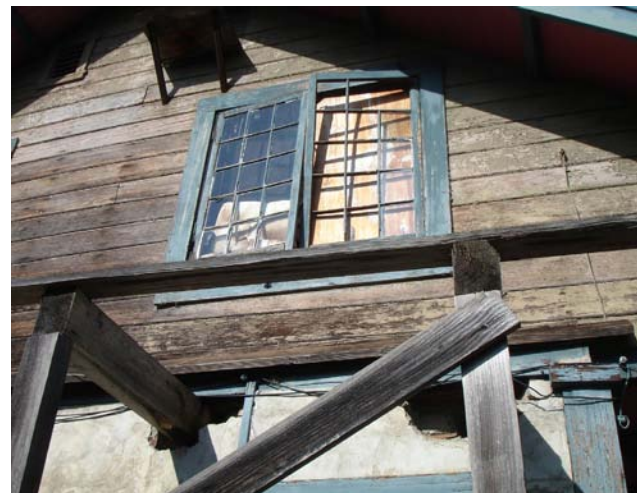
Recent photo of Briones house showing how house is left open to the elements. (Courtesy M. Blum)
